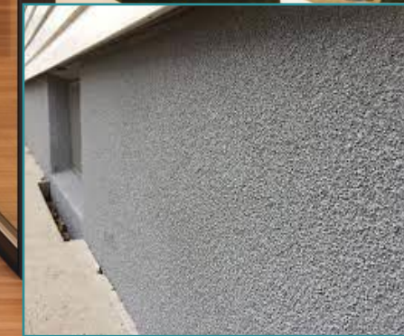
Thermal Protection Roof & Walls
